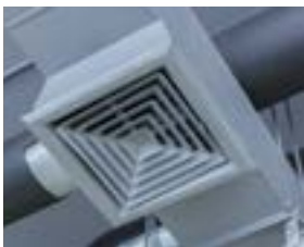
Ventilation duct monitoring
